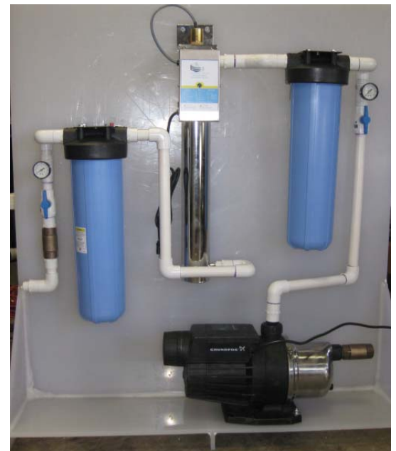
Rainwater Treatment Equipment
